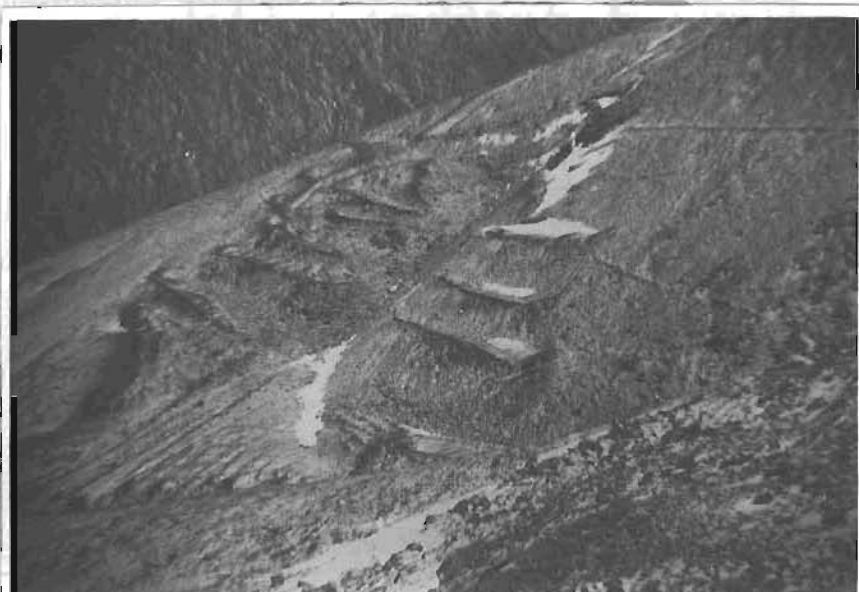
Figure 8. View of excavation work from a point on the east side of the bulldozer cut.
