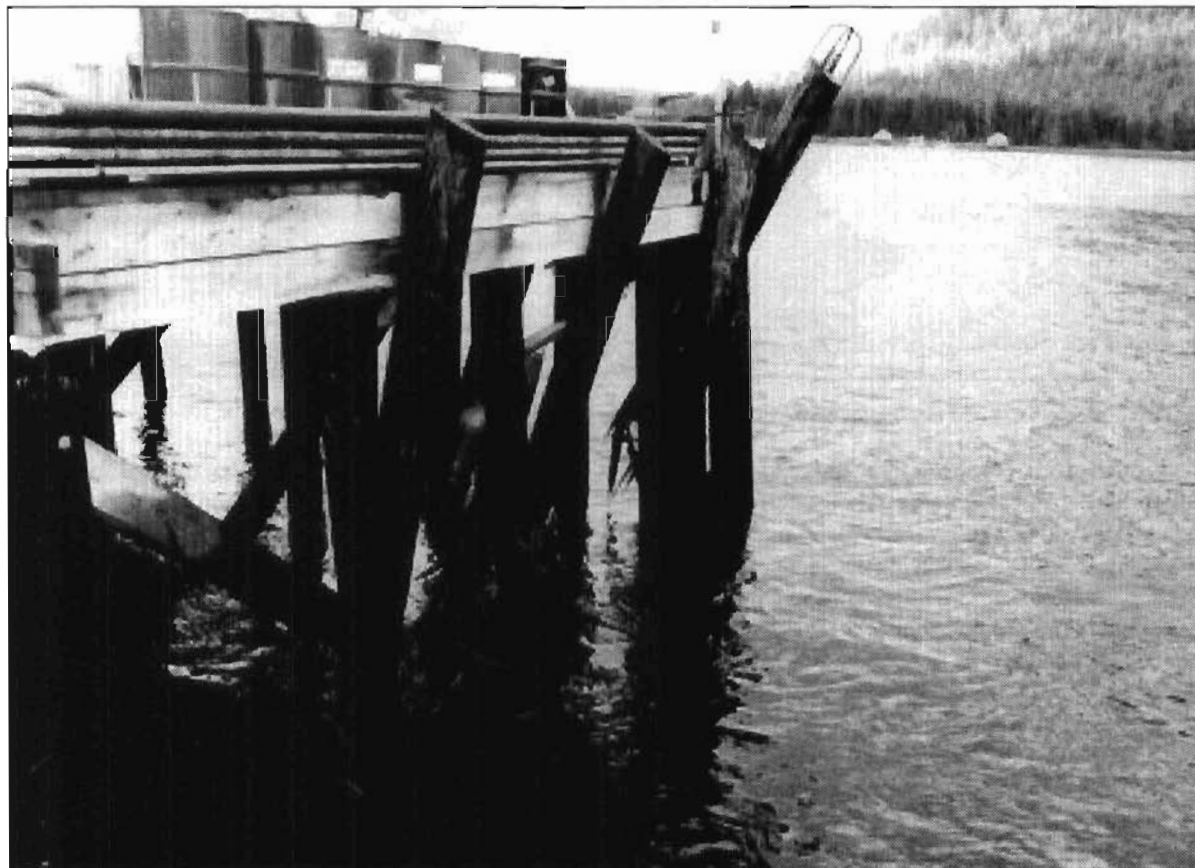
Figure 4. Pilings snapped by tide-driven iceberg at Petersburg fuel dock.
