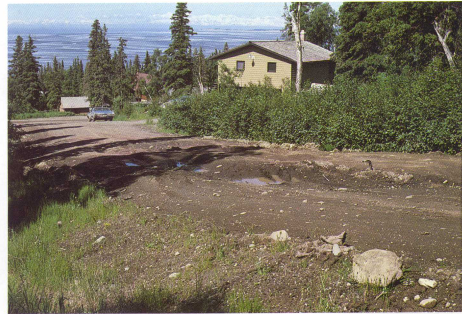
Figure 3a. -- Road damaged by seepage of shallow ground water (172nd Avenue near Goldenview Drive, June 1979).
