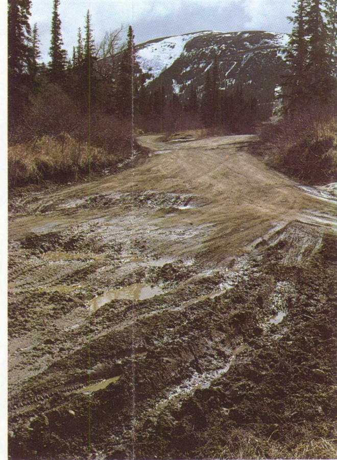
Figure 3d. -- Road damaged by poor drainage and high water table during the spring (Carl Street near upper Little Rabbit Creek, May 1980).
