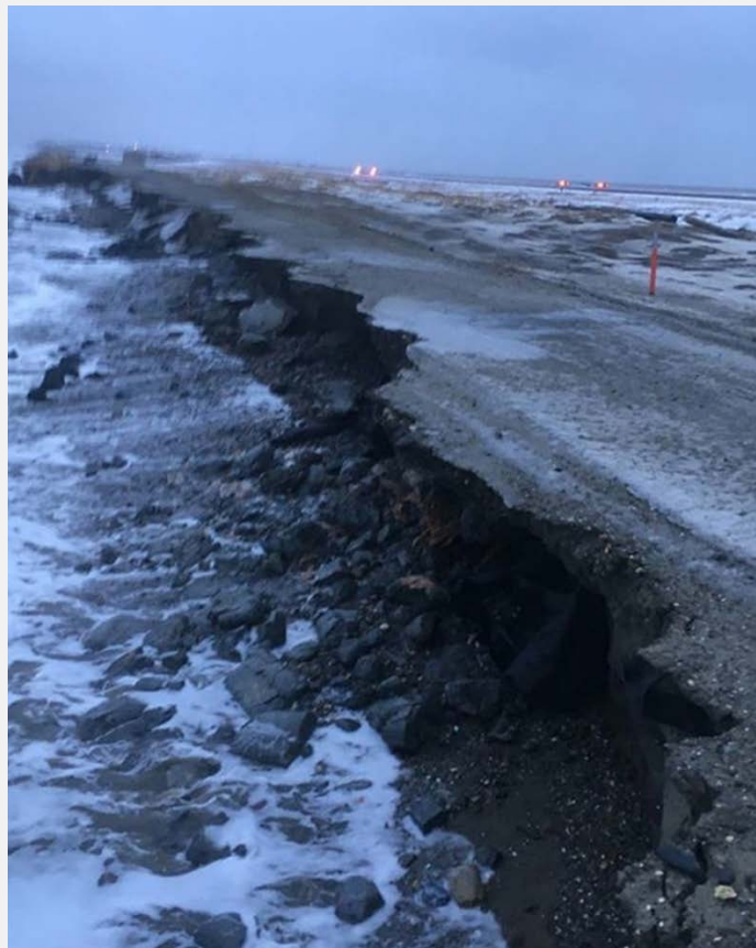
Figure 8: Erosion at the landfill access road, photo taken by the Native Village of Shishmaref after November 2017 storm.
