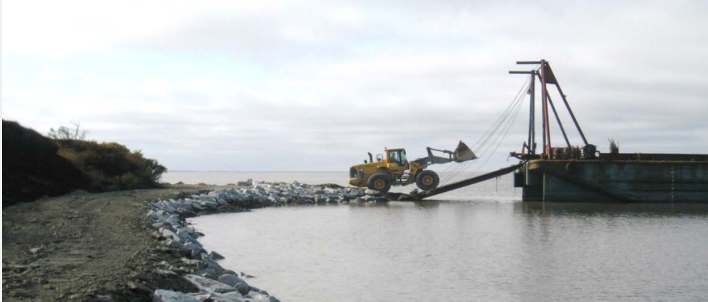
Figure 3: Heavy equipment loading the last seasonal barge in Mertarvik, after completion of the beach road to the barge landing. Photo taken by Robert Lundell, Alaska Department of Transportation, 2009.
