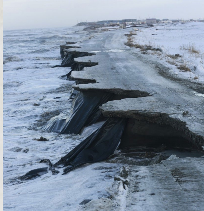
Erosion at Shishmaref, Nov 2020 Twyla Thermond, Native Village of Shishmaref
