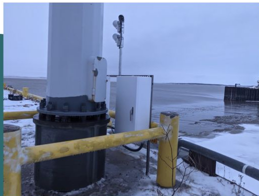
Dillingham City Dock Bubbler Water Level Station 2022 (photo courtesy JOA Surveys)
