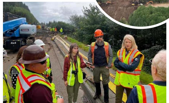
Officials, including Senator Lisa Murkowski, visit the site of the August 27 landslide in Ketchikan. Photo: Michelle Kubalack. Inset. Aerial view of the landslide. Photo: Lance Kramer.
