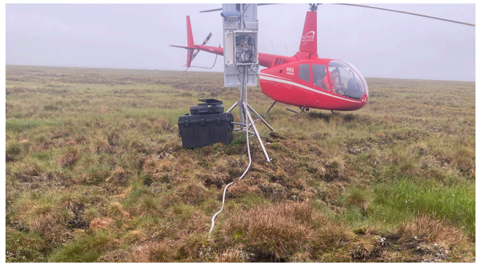
Radio repeater site on the North Slope. Repeaters are a critical tool in remote fieldwork that allow staff to communicate with one another.
