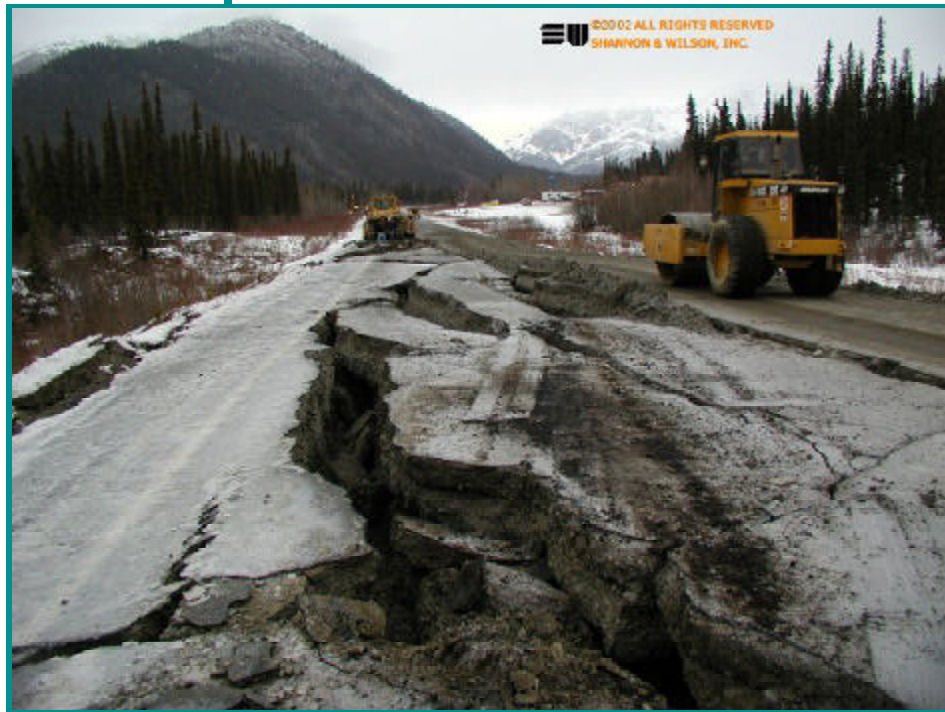
Road surface at Milepost 78 along the Tok Cutoff, showing damage from the magnitude 7.9 Denali Fault earthquake of November 3, 2002—the world's largest earthquake of that year. View looking north towards Mentasta Lodge on the east (right) side of road shows approximately 4 feet of vertical and 6 feet of horizontal displacement across the road. Photo provided by Shannon & Wilson Inc. from Web site ( http://clients.shanwil.net/project.php?projectid=Fairbanks_Quake_2002 ).
