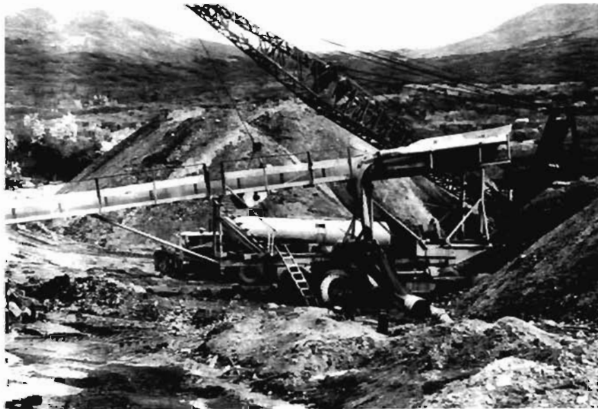
Fig. 4. Side view of sluicibox. Note fuel storage tank in background. Flat Creek Placers.
