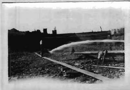
Hydraulic lift, Donlin Creek.
