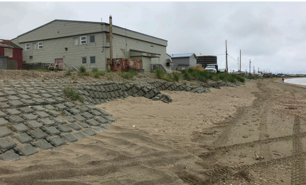
Figure 12. Erosion control structure at Deering, which was undermined and damaged by storm surges. Photo taken July 2018.
