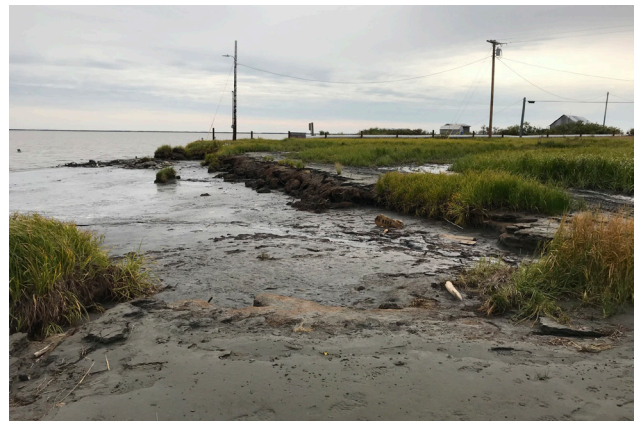
Figure 17. Erosion at Nunam Iqua near power poles and community water source intake pipe. Photo taken August 2019.
