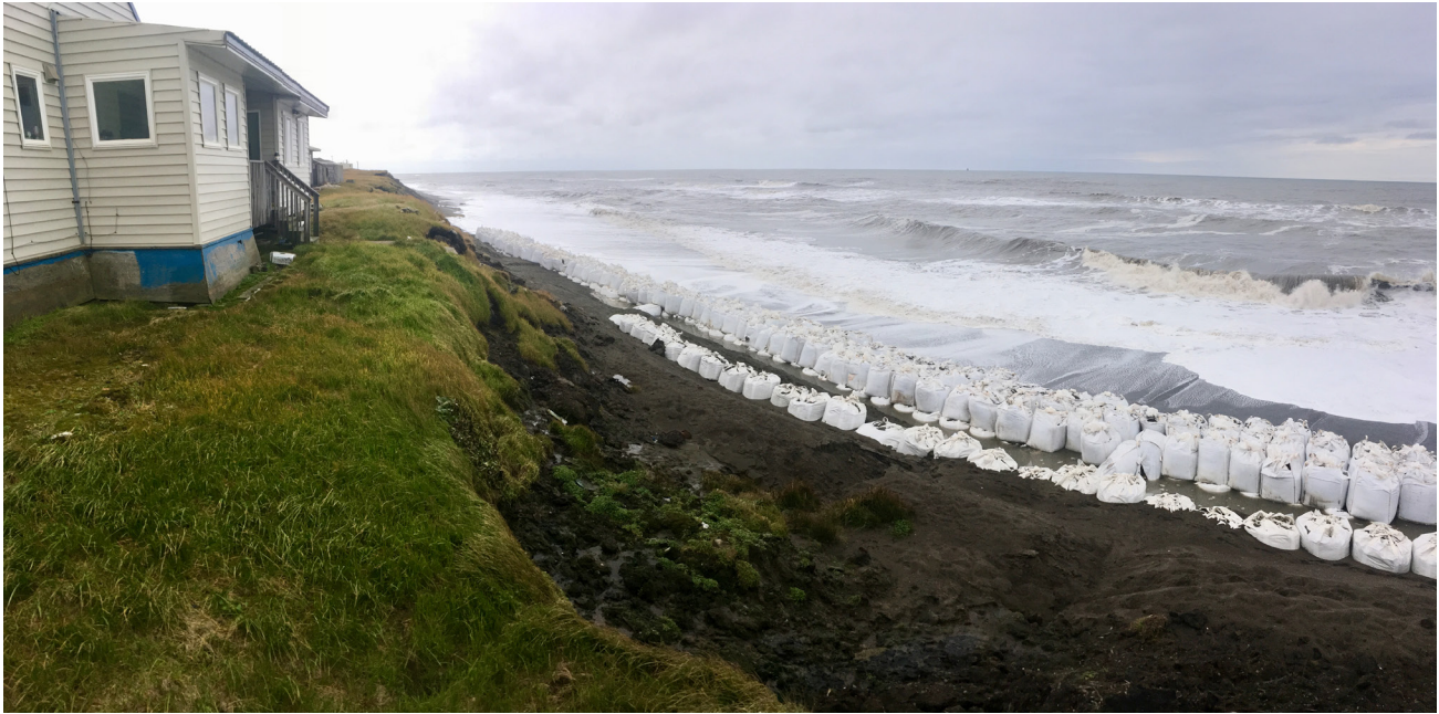
Figure 6. Erosion of ice-rich coastal bluffs at Utqiagvik during a coastal storm. Photo taken August 2019. Sandbags have been placed at the base of the coastal bluff to mitigate erosion.
