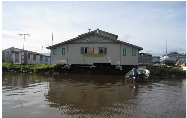
Figure 18. Building overhanging river bank at Kotlik. Photo taken June 2017. Concrete blocks from dilapidated NRCS erosion-control structure piled along river bank.
