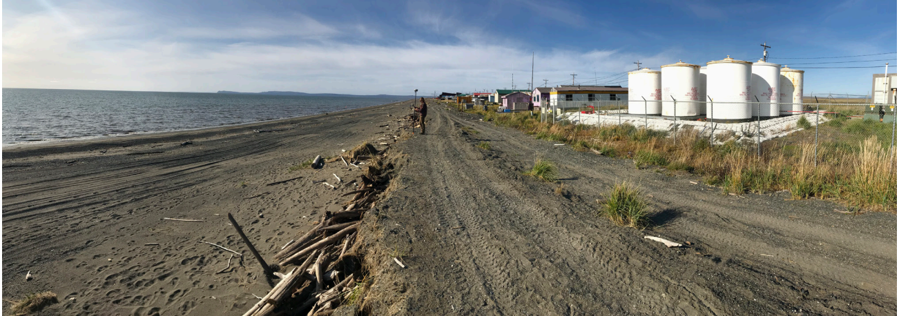
Figure 13. Unconsolidated gravel berm (used as a road) in front of the tank farm in Shaktoolik. Photo taken after a storm in August 2019 eroded the berm.
