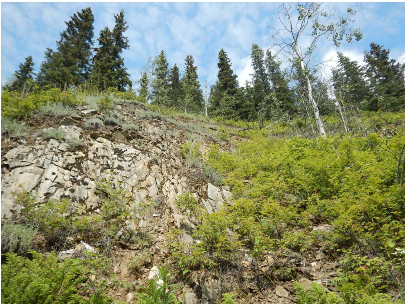
Figure A41. Image of BigB5_7S_6E_24_SW1 from July 1, 2020. This view is looking upslope at the head scarp region and exposed bedrock outcrop. Photograph taken by MD.
