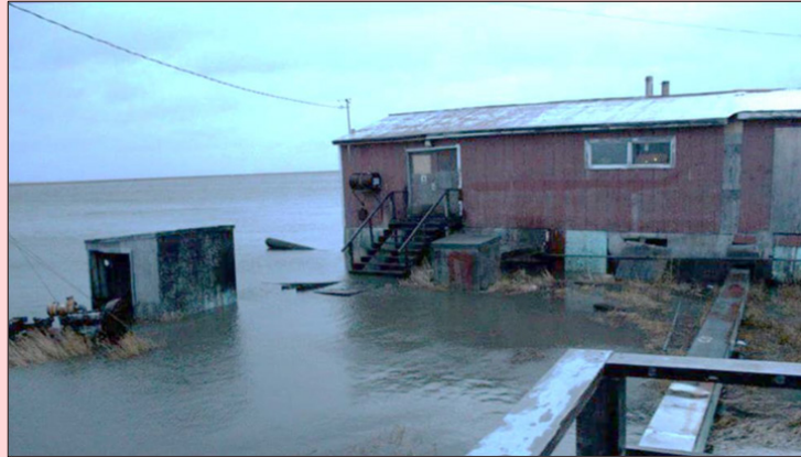
Figure 1. Flooding at Head Start utility building on October 5, 2017, in Chefnak, Alaska (PND, 2018).
