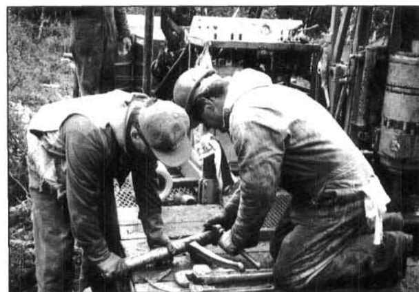
Figure 13. Mark Musial of Golder and Associates and Ken Elordi of Boyles Brothers remove a split spoon sampler from a drill during tests of a proposed tailings dam site at Nixon Fork project near McGrath. (Photo by Richard Flanders)
