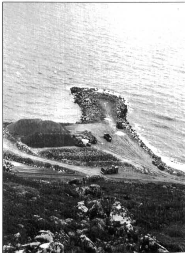
Figure 15. Sound Quarry Inc. crew constructs a causeway for riprap shipments to various Bering Sea villages at the company's Cape Nome Quarry about 15 miles (22 kilometers) southeast of Nome. (Photo by T.K. Bundtzen)
