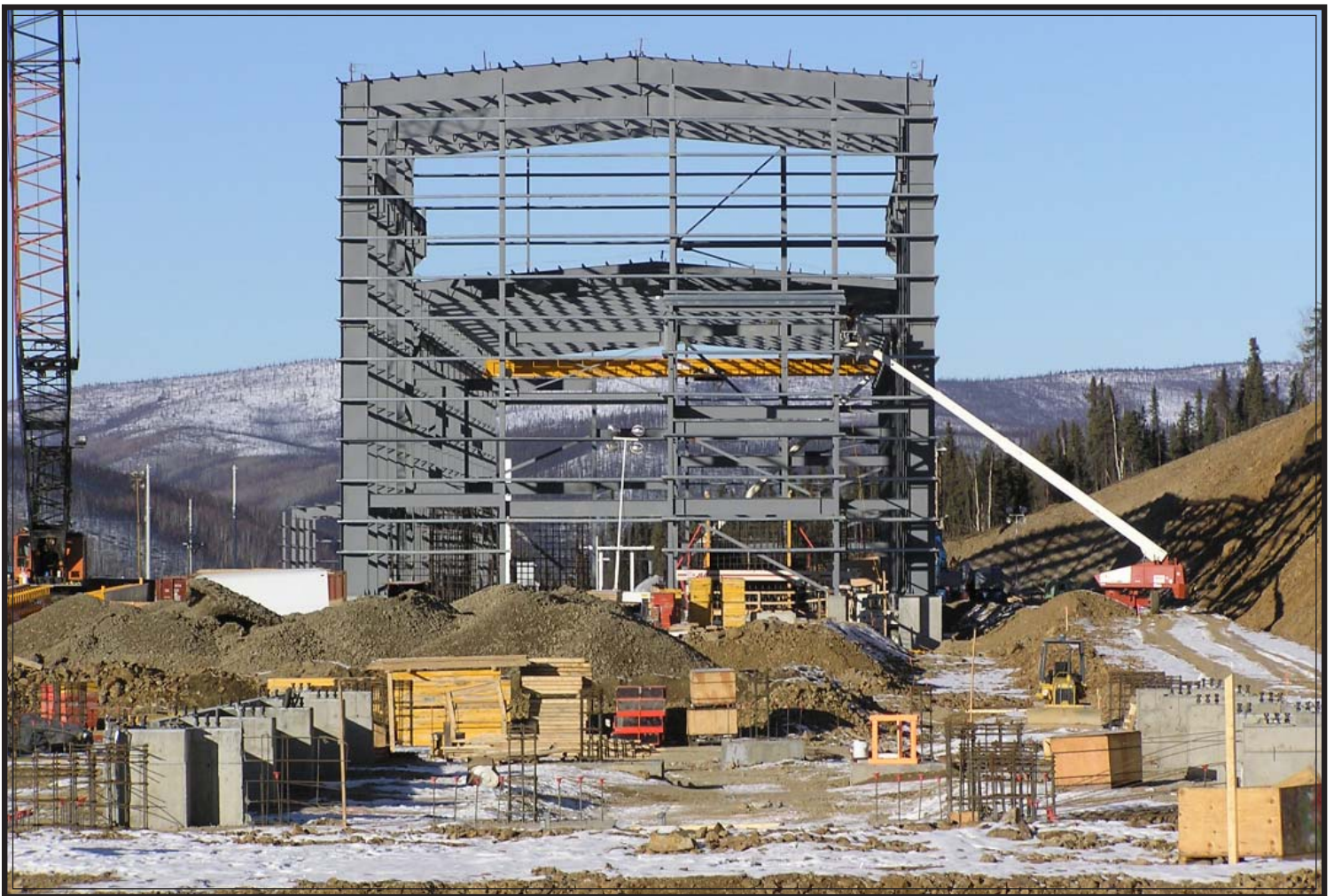
Construction of mill facilities at the Pogo gold project. The mill bench was leveled by May 2004, first steel was erected on the mill building in August 2004, and interior concrete work began late in 2004. Photo provided by DNR-ML&W.
