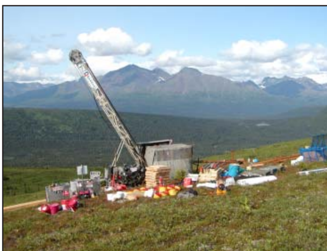
Figure 15. A NANA–Dynatec Drilling LLC LF-70 core drill rig onsite in the Alaska Range near the Rainy Pass Lodge. Photo by Russ Franklin, Kennecott Exploration Co.
