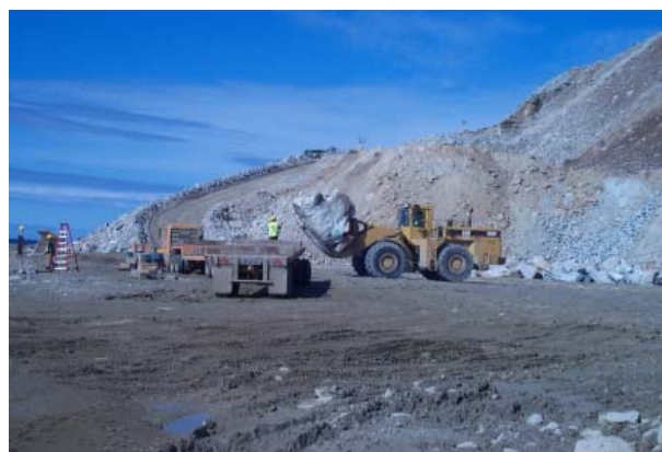
Figure 30. Loading granitic orthogneiss boulders on semi trailers at the Cape Nome Quarry. The rock is trucked to Nome for use in stream bank armoring, seawall construction, and other projects in Nome and other communities on the Seward Peninsula. Photo by David Szumigala.
