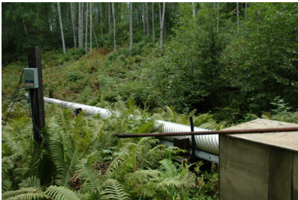
Figure 12. Well, Pump and Pipeline at Hetherington Property
