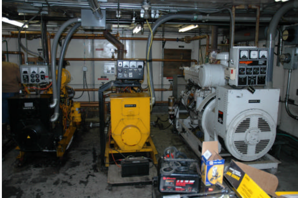
Figure 11. Diesel Generators at Power Plant
