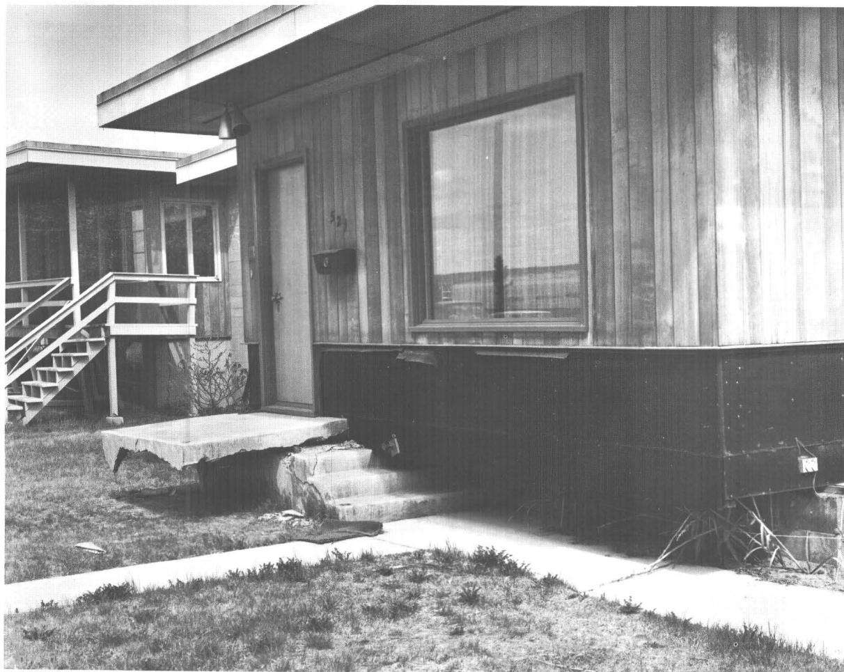
29.—House pushed off foundation by pressure ridge at toe of L Street slide. Well-framed house not otherwise visibly damaged. Push must have been shallow and nearly horizontal.
