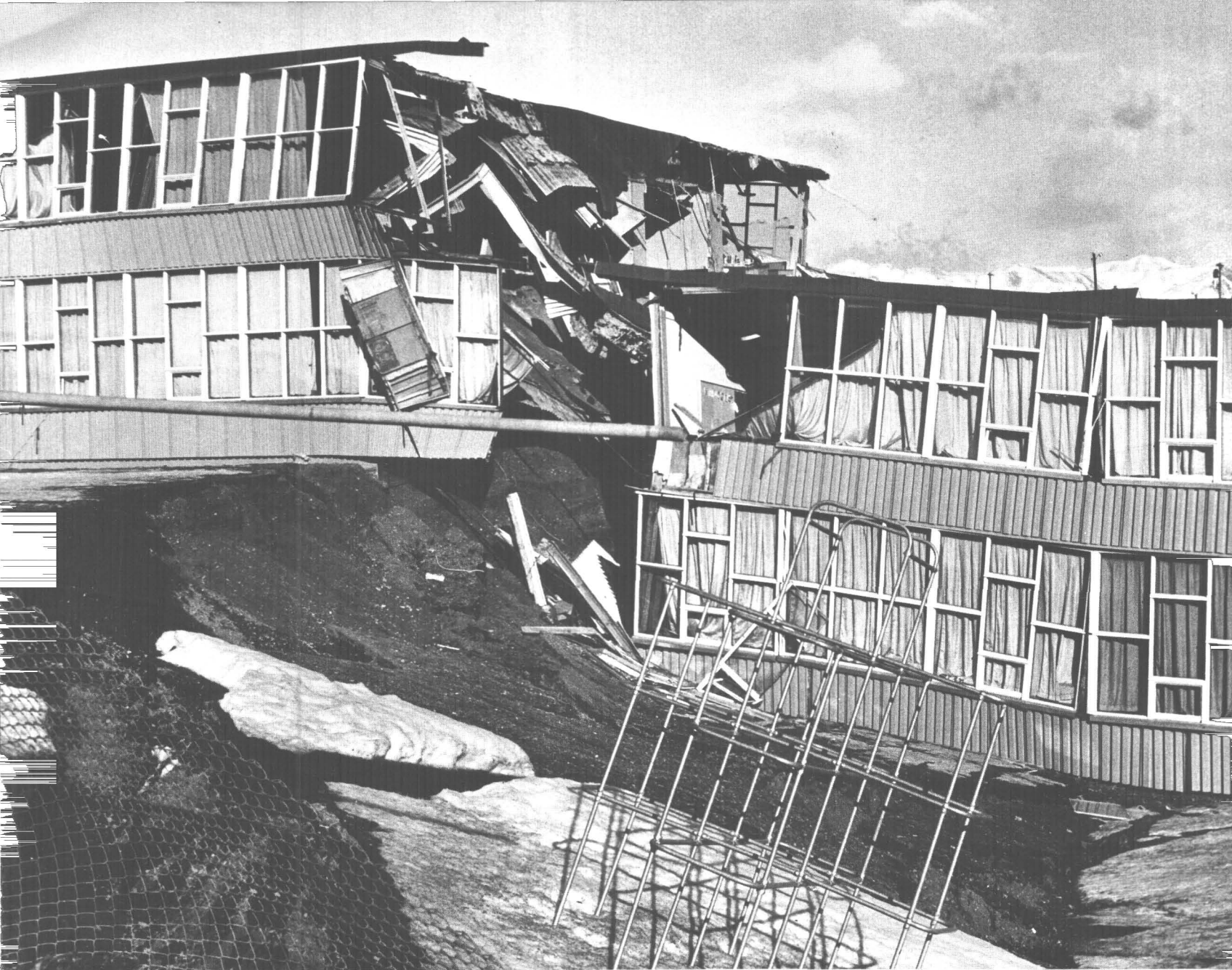
3.—Wreckage of Government Hill School. The south wing of the building, shown here, collapsed into a graben at the
