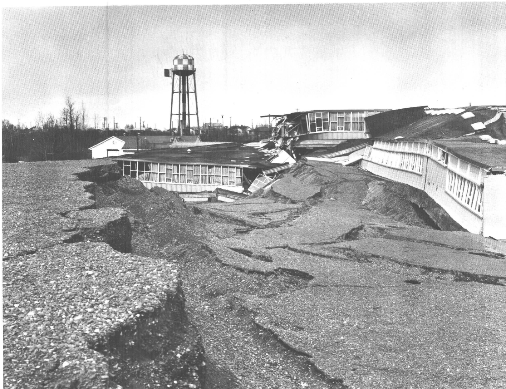
36.—Wreckage of Government Hill School as viewed from the playground, looking west. Graben in foreground is about 12 feet deep. Note undamaged water tower.
