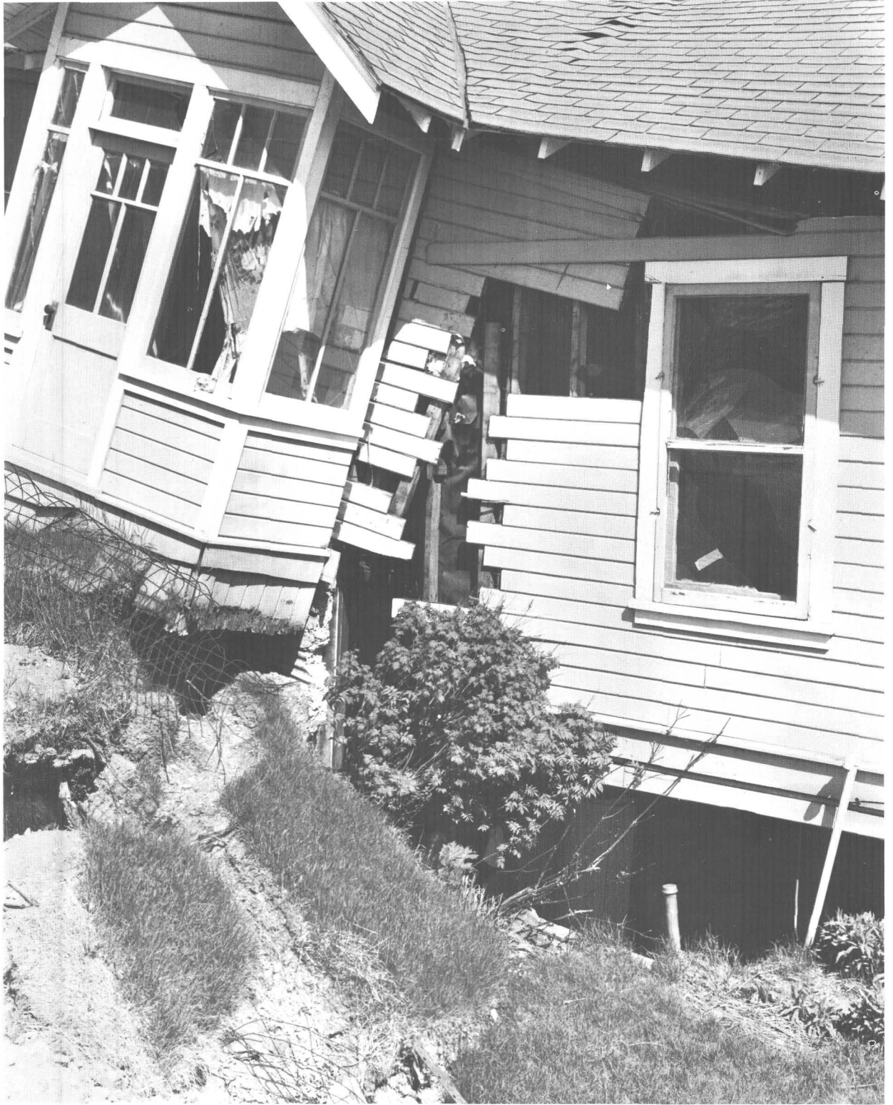
28.—Wrecked dwelling astride bounding fracture, L Street graben at Eighth Avenue and N Street. Damage caused entirely by ground displacement along fracture.
