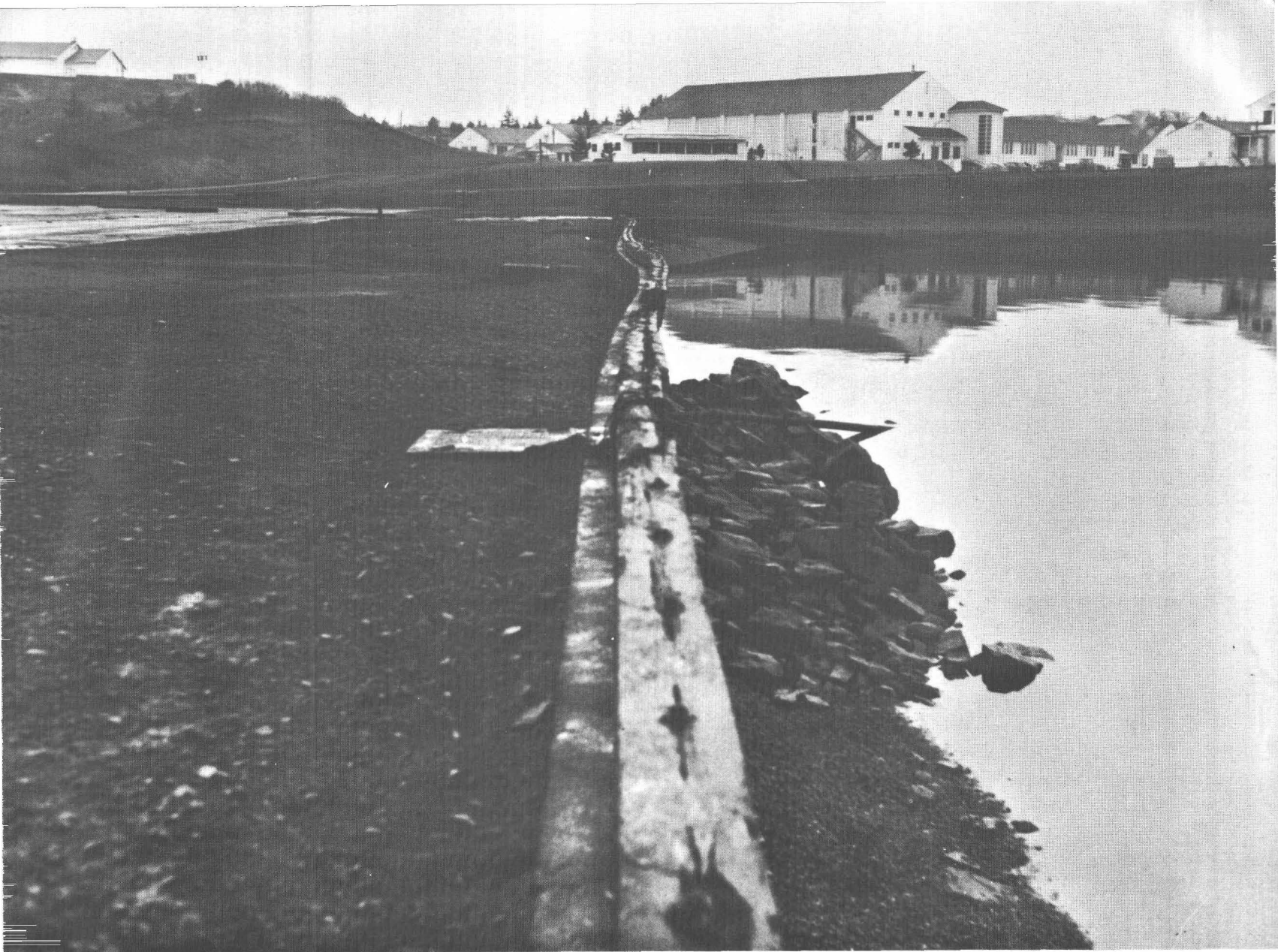
4.—Displacement of seawall toward Womens Bay, Kodiak Naval Station. View is east. Photograph by U.S. Navy, April 1, 1964.
