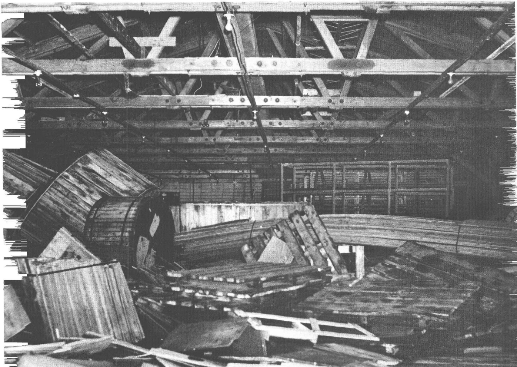
13.—Photograph of interior of supply building, Kodiak Naval Station, showing condition of supplies stored in building after the retreat of the seismic sea waves. Photograph by U.S. Navy, March 29, 1964.
