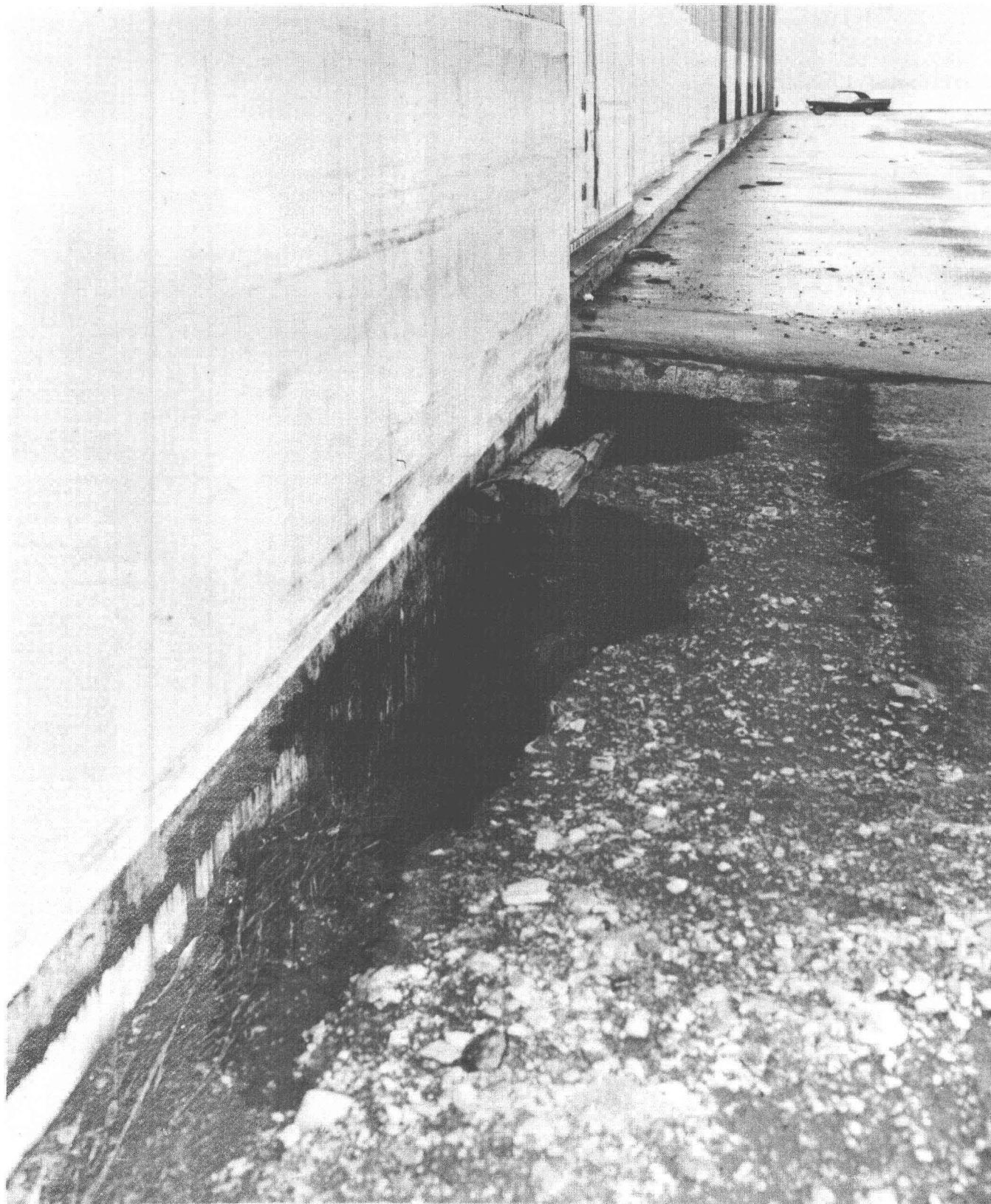
5.—Result of compaction of fill debris underlying asphalt aircraft ramp outside hangar at Kodiak Naval Station. Note the settlement of back-fill material adjacent to foundation of structure in the foreground. Photograph by U.S. Navy, March 29, 1964.
